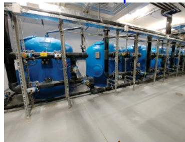
Multimedia filtration system
